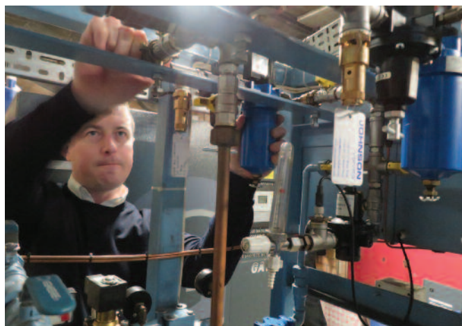
Stephen Hutchings servicing a medical dryer.
